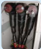
example of sensor installation
