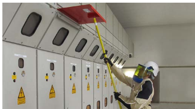
Inserting an insulating protective shutter (type A3) by means of an operating stick
