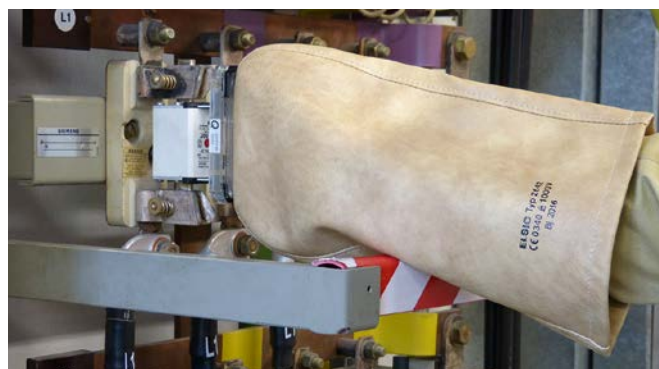
Operating an NH fuse with an NH fuse handle with sleeve.
