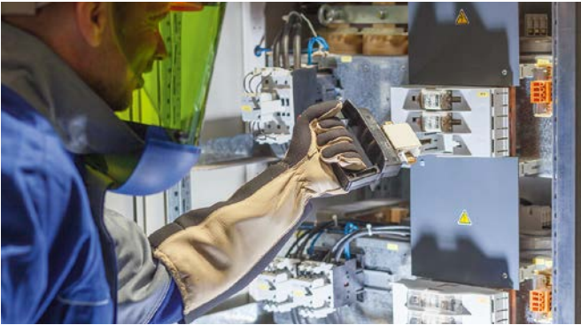
Actuation of an NH fuse puller using protective gloves.
