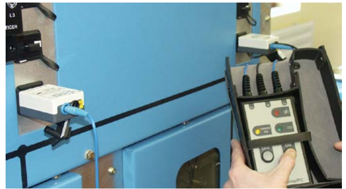
DEHNcap/PC-LRM phase comparator with two HR-LRM test adapters used in an HR switchgear installation
