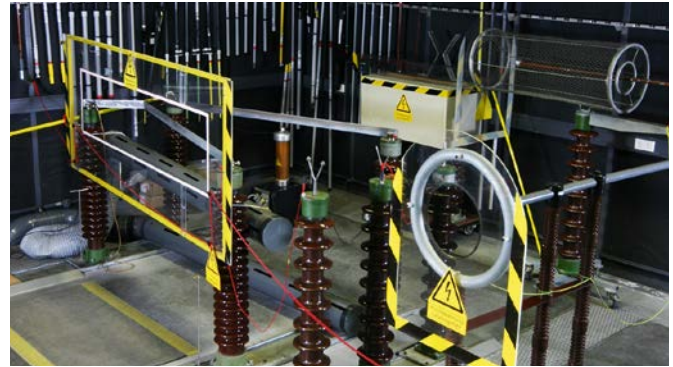
One of our high-voltage laboratories.
