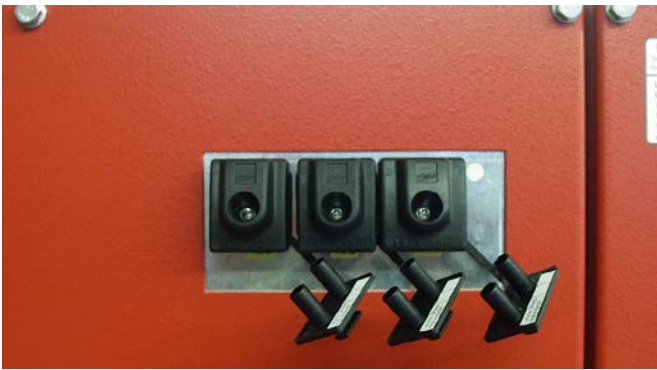
DEHNcap/P passive voltage indicator used in an encapsulated switchgear installation.
