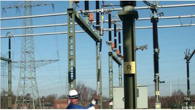
Use of an ASP distance voltage detector in an outdoor switching station
